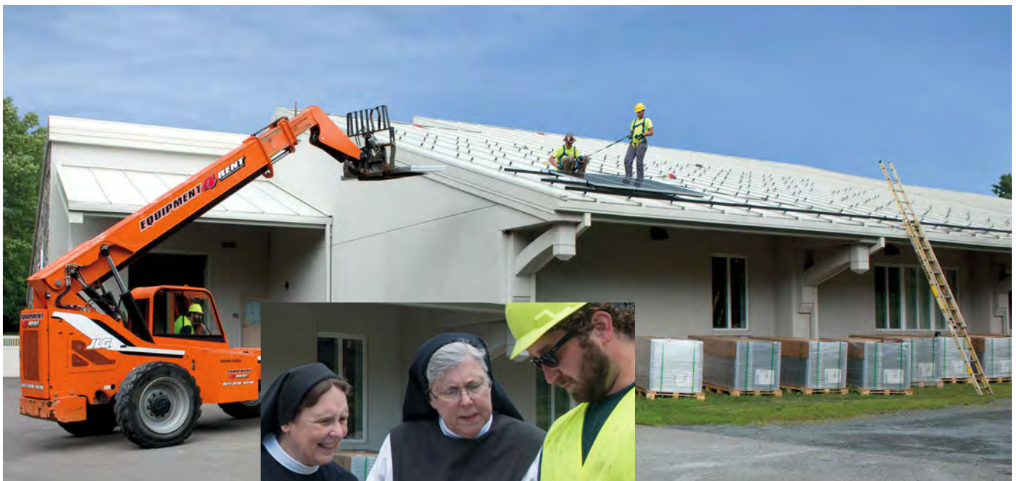
A 2016 NRRO Implementation Award underwrote the installation of solar panels, which will drastically reduce energy costs. From left: Abbess Mother Maureen McCabe and Sister Mariann Garrity discuss plans with Derek Sabin, construction manager for Suncommon, a company that specializes in solar-energy solutions.
