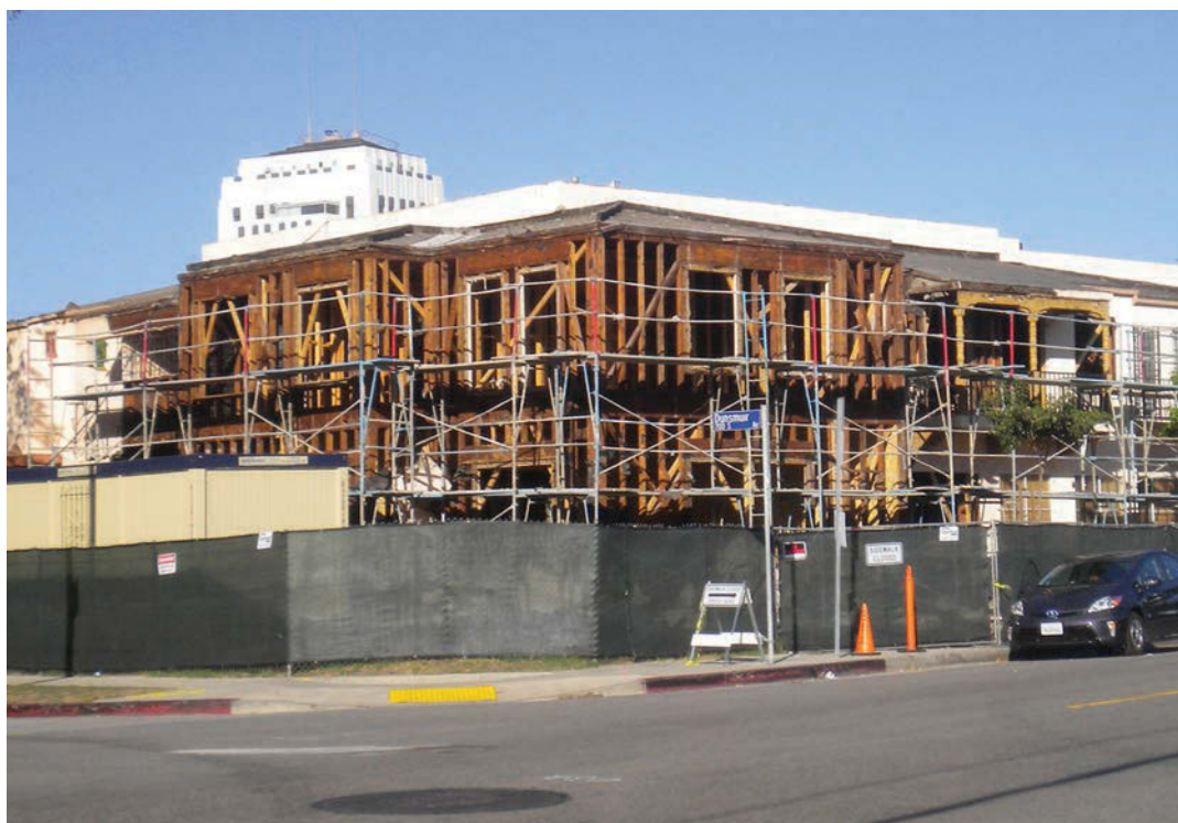
Left: Shown during demolition in 2015, the community's provincial house was built in 1930. It needed to be expanded and renovated to provide elder-friendly space for senior members.
